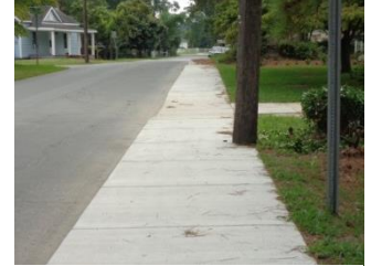
New sidewalk on Barden Street connects Fayetteville Street to the Sampson Center.
